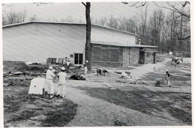
Carpenters and Cement Masons working on a project (renovation of the gym).
