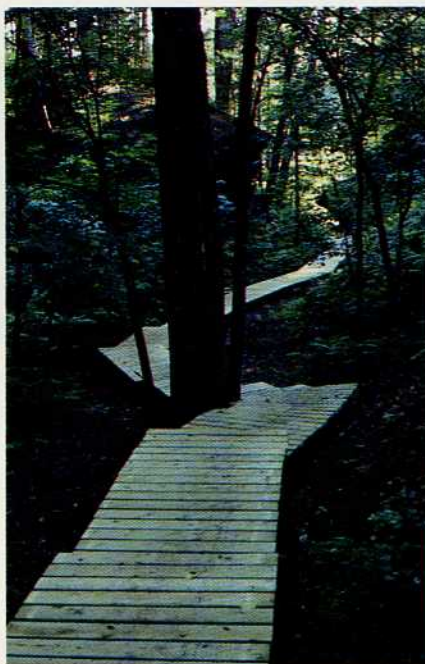
WCC built this eye-catching, meandering trail at Blackhawk Island Natural Area in south central Juneau County. Visitors used to slog through wet soils, dampening their sneakers and trampling rare plants in Spring Gulch. Now, everyone is happy.
