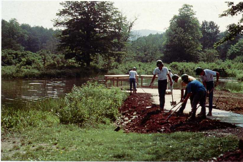
Corps members put finishing touches on a handicapped-accessible fishing platform in Allegany State Park.
