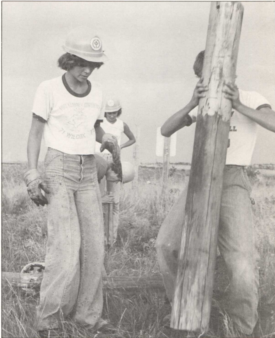
These workers are helping construct a hunter access parking lot in Nebraska.
